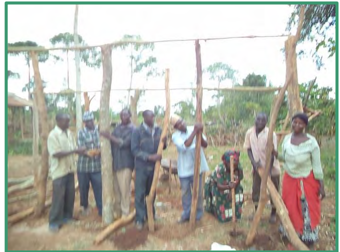
A FFLG IS WORKING TOGETHER TO CONSTRUCT A GOAT SHELTER FOR ONE OF THE MEMBERS
