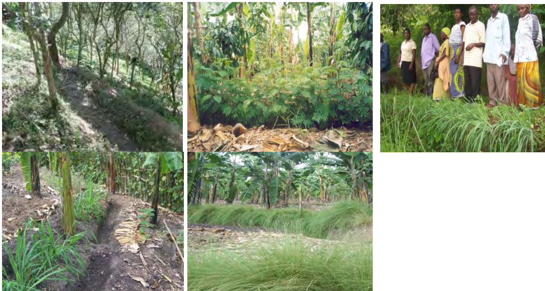
Trench digging (and planting stabilizer grass or shrubs on edges) to prevent soil erosion
